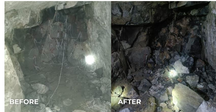
Controlled blasts using pyrotechnics to advance over 1 m each time in the Bonanza galleries (Mar-26)
